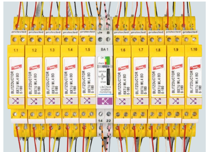
Installed DEHNrecord condition monitoring system
