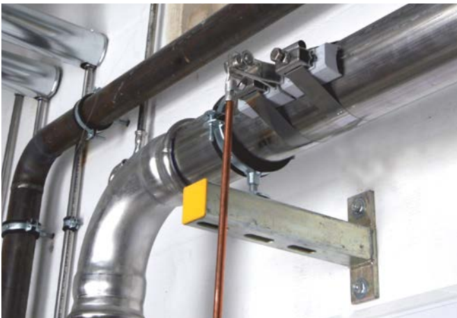
Installed at a StSt pipe.
